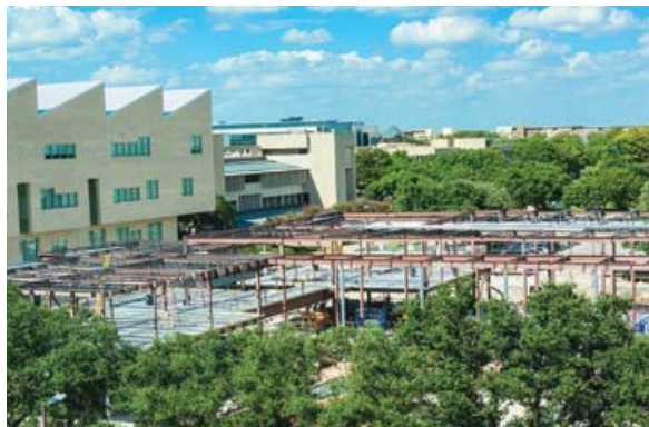
Left: Construction on the center as of September. Visit alumni.utdallas.edu/davidson-gundy-alumni-center for a livestream of the progress.
